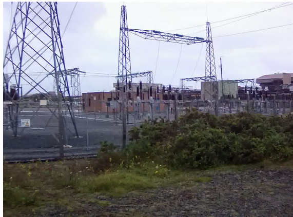
Photo 1: Aughinish Alumina works with the ESB Sub-station.
