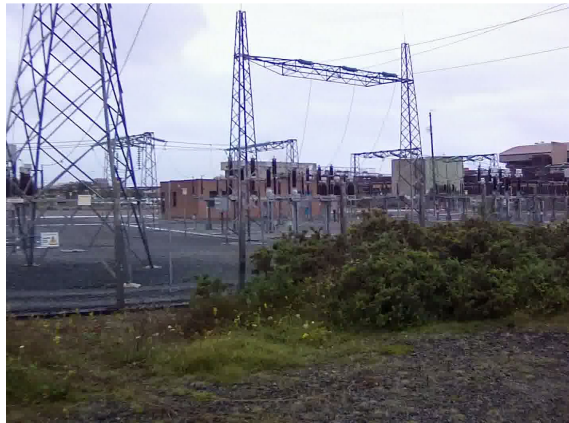
Photo 1: Aughinish Alumina works with the ESB Sub-station.
