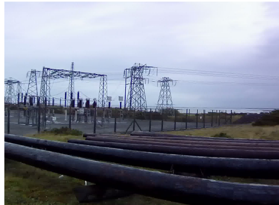
Photo 2: ESB 110kV Sub-station located well above high tide levels, at the southern end of the site.
