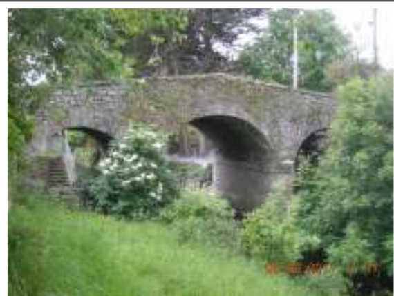
Photo 4: Three arch bridge. The left hand arch is blocked to around half of its height and the right hand arch is partially blocked
