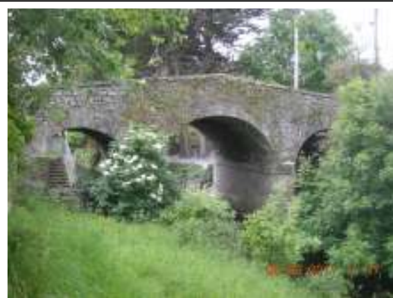
Photo 4: Three arch bridge. The left hand arch is blocked to around half of its height and the right hand arch is partially blocked
