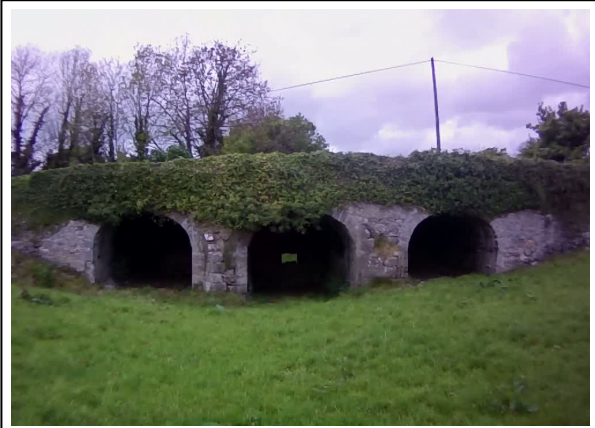
Photo 2: Overflow arches at the Clodiagh River Road Bridge in Rahan, blocked up.
