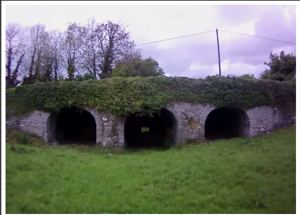
Photo 2: Overflow arches at the Clodiagh River Road Bridge in Rahan, blocked up.
