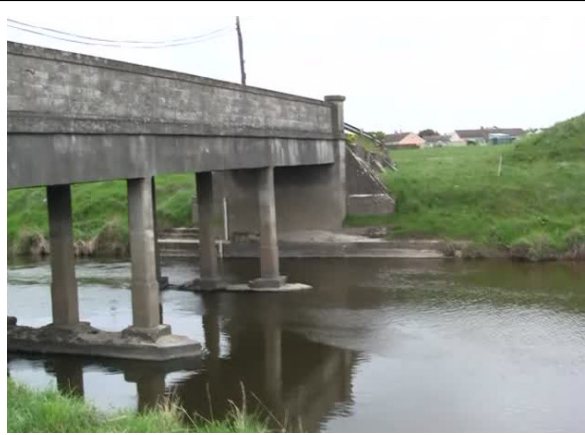
Photo1: Upstream face of bridge over the River Brosna at Pollagh. Properties at risk in the background.
