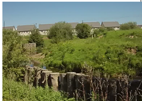
Photo 4: Timber piles protecting against erosion, downstream of the confluence.
