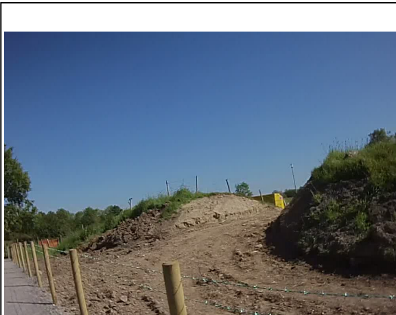
Photo 2: Gap in left bank embankment near the industrial estate.
