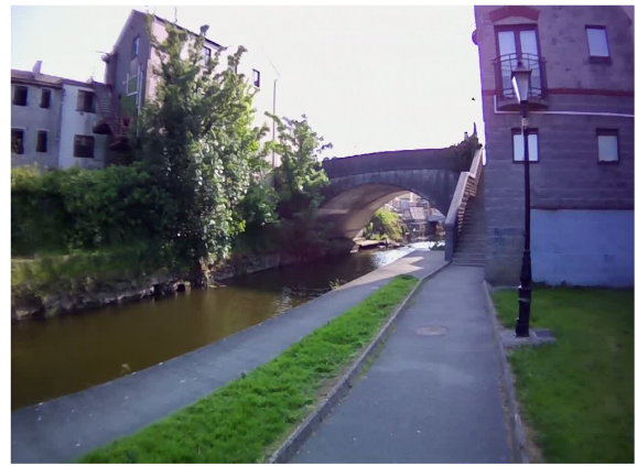
Photo 2: R198 road bridge over the River Camlin, viewed from the upstream right bank.
