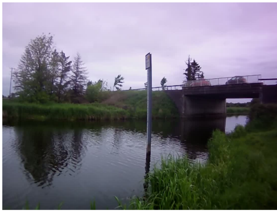
Photo 1: N5 road bridge over River Camlin upstream of village viewed from upstream right bank.
