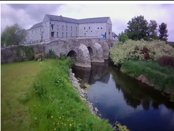
Photo 3: Former mill buildings and minor road bridge, viewed from the upstream left bank.
