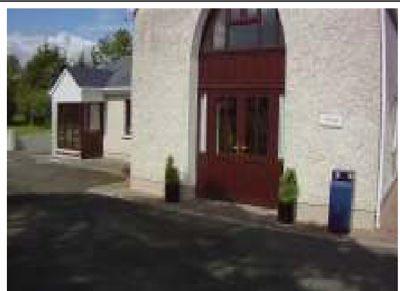
Photo 4: Emmanuel House of Providence shop building. Note the newly constructed flood wall at the rear of the building.
