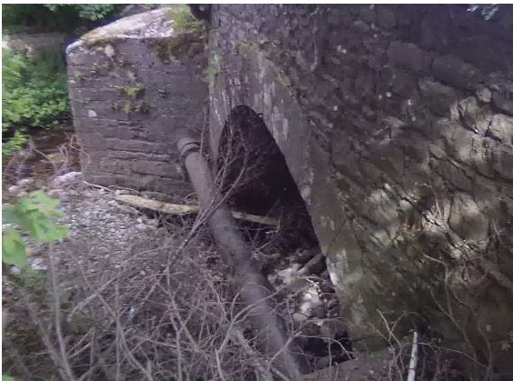
Photo 3: Upstream face of Main Street bridge over Gorragh River from the right bank.
