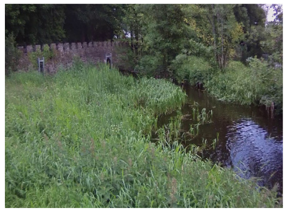
Photo 2: Flood gates installed at culverts beneath access roadway to Island House.
