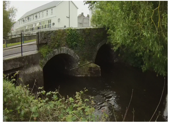
Photo 2: Bridge Street bridge over the River Camcor from the upstream left bank
