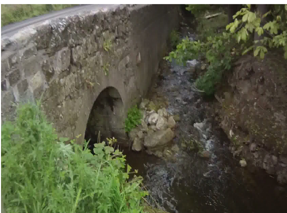
Photo 3: Confluence of tributaries to the River Inny, flowing parallel to and under the N55 north of the town centre.
