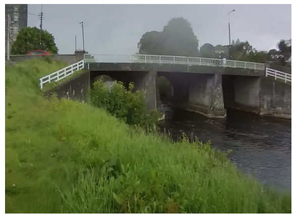
Photo 2: N55 road bridge over the River Inny from the downstream right bank
