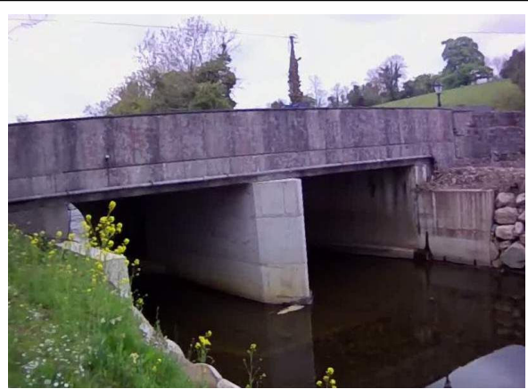
Photo 2: Upstream face of bridge where flooding on the right bank has occurred in the past
