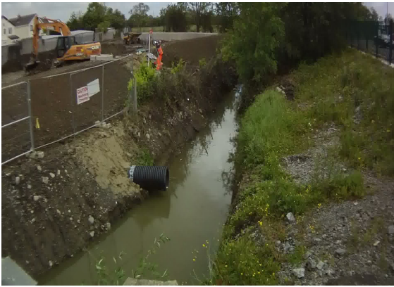
Photo 1: Looking downstream of the road bridge adjacent to the OPW flood alleviation scheme (nearing completion) in the upper section of Ballinasloe.
