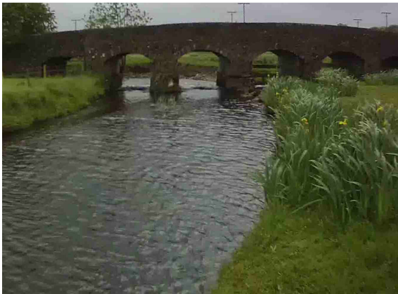
Photo 1: Main road bridge over the Ahascragh River looking downstream from the right bank.
