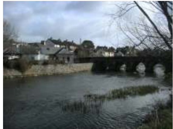
Photo 2: Downstream side of multi-arch bridge. Some low properties on d/s side on right bank.
